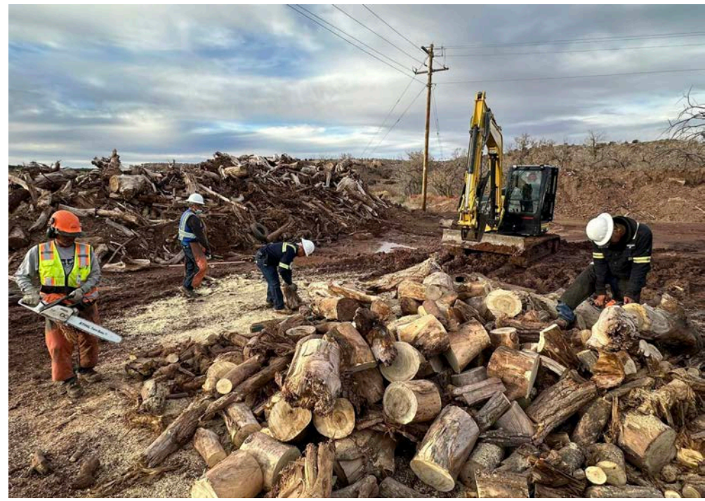
PHOTO - Wood pile for Project Chizh for Elders located adjacent to the new hospital.
